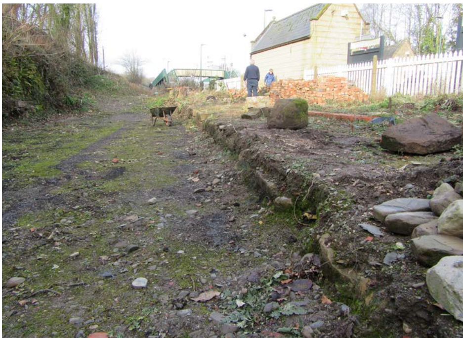
More of the original platform edge is slowly being revealed, and the condition of the stones uncovered so far is largely very pleasing
