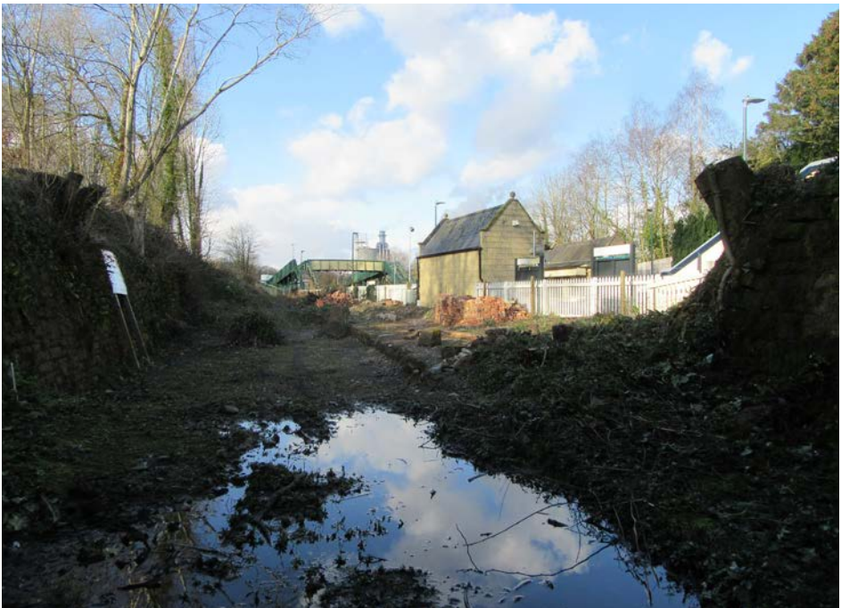
There was certainly some heavy rainfall in February - taken from under Hand Lane bridge, this shows an area we clearly need to keep an eye on.
