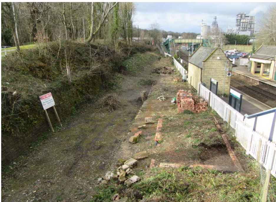
How the site looked at the end of what would turn out to be the last working party before the Coronavirus lockdown period.
